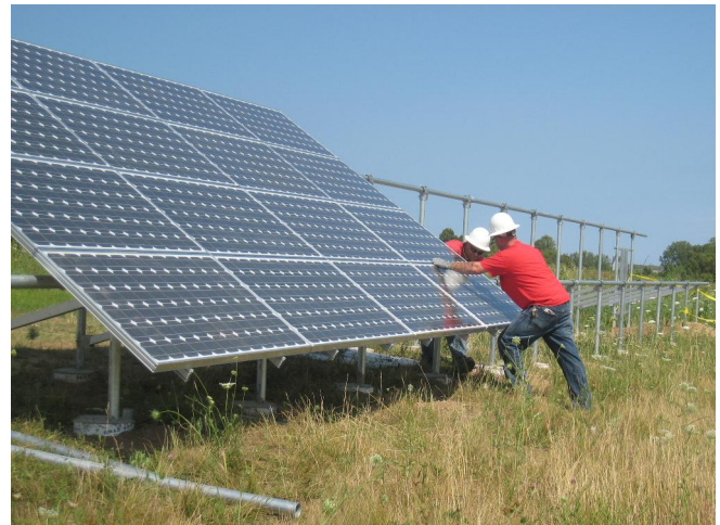
Solar panels now supply electricity to the Education Center
